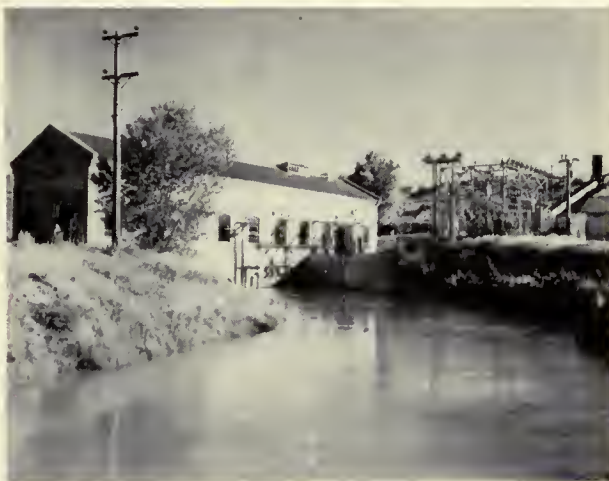
"ELECTRICITY FOR MILES AROUND."—The Lingle power plant, one of the first built by the Bureau of Reclamation, astride the Fort Laramie Canal which supplies irrigation water for the south side of the Platte valley. Photo by Norton T. Novitt, Region 7.
